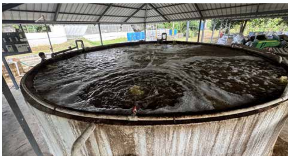
Close view fo bio-digester
